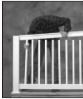
Position top rail over balusters. For convenience, rest the high end of the rail on the next post.
