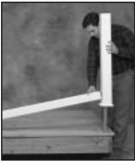
Lift next post and insert rail into opening. Push post and rail down to deck.
